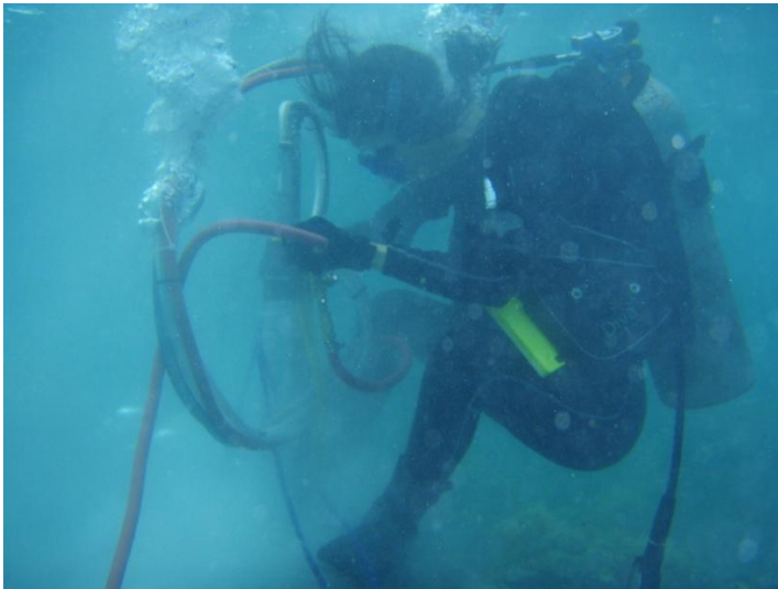
Figure 21. The operation is simple and easy. No training is necessary. The drill goes down on its own, so the operator only needs to hold the drill. Extra pressure from the driller will speed up the drilling. Water gets cloudy from the drilling debris.
