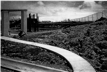
Figure 3.17. Erosion and scouring caused by "green" sea water being forced more than 80 feet up the face of a cliff at the South Tipalao housing area, Orote Peninsula, Naval Activities, Guam.
