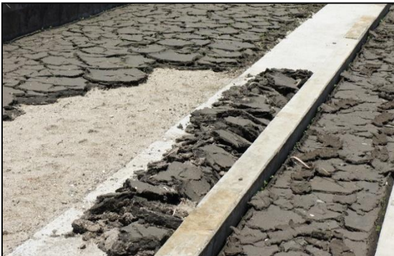
Dried sludge at the Yap Wastewater Treatment Plant
